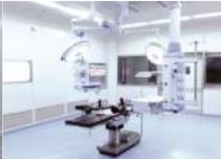
Integrated purification for operating room
